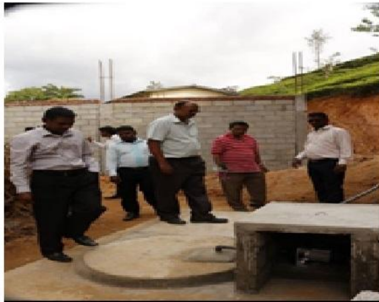
IMHO Board members visited the area and inspected the newly installed school water system in Maskelia.
